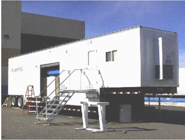
(a) System installed at RFETS site
