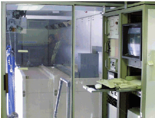
(c) SuperHENC and Control Cabinet
